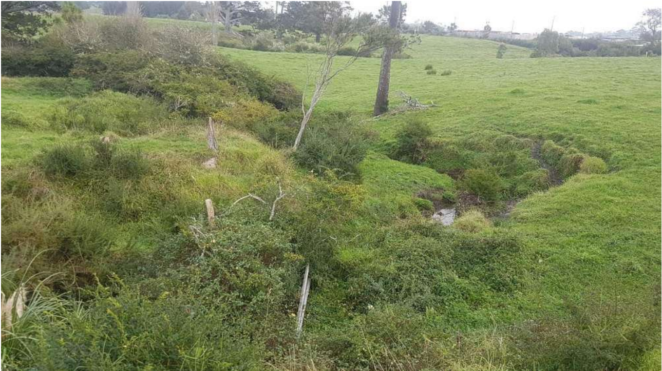
Photo 6: Dairy Stream viewed from Dairy Flat Highway showing stream bank erosion/slumping within the Structure Plan Area
